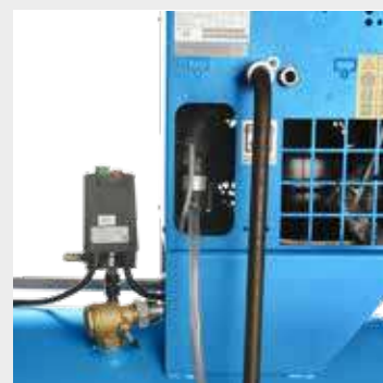
Pre-installed and connected
