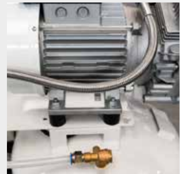
Pump unit mounted on anti-vibration devices
